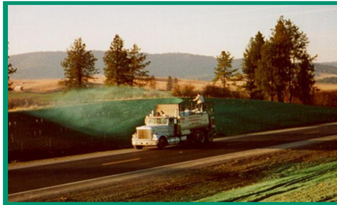
Hydroseeding project demonstration on Highway 9 between Deary and Princeton: a slurry of native plant seed and wood fiber mulch.
