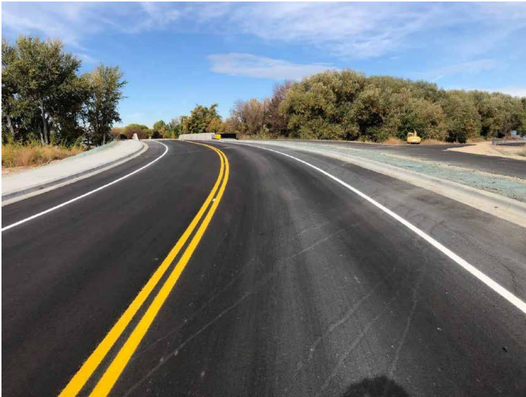
Continuing North Moving into Phase I – Willow Creek Bridge and Middle School Access (right)
